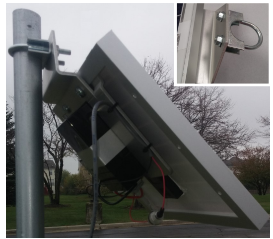
Figure 2: Solar Panel connected to post
