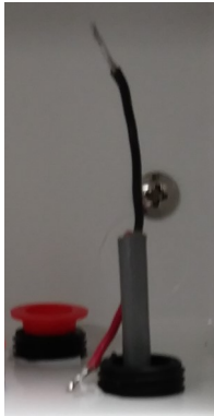
Figure 3: Power cable through gland
