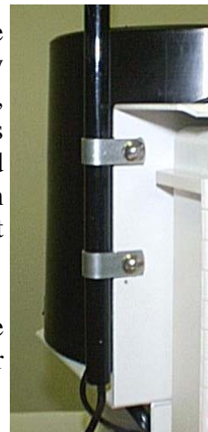
Anemometer clamped to back plate
